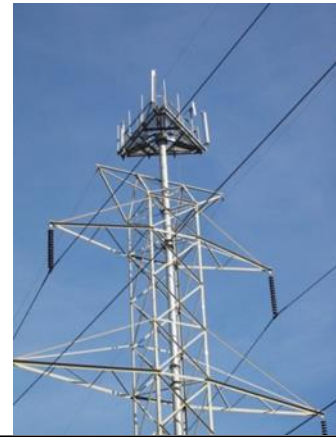
Photograph of a Ft. Worth Attachment. Source: http://www.bge.com/doingbusiness/li ghtspeedcommunications/PublishingImages/Main/Fort%20Worth.JPG
