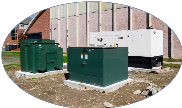
BRIC Funding was used to install this generator at East Stroudsburg University
