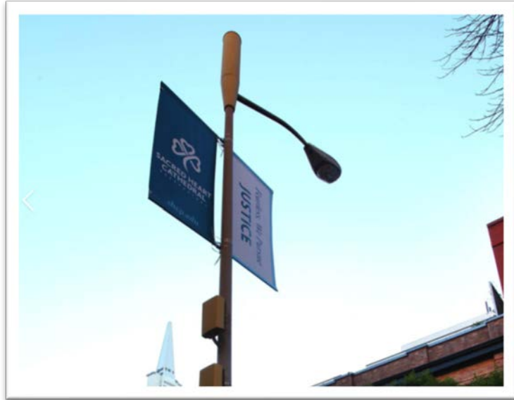
Example of a Small Wireless Facility
