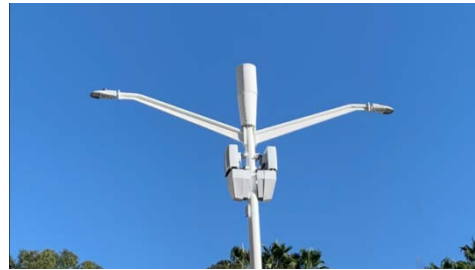
Another example of a Small Wireless Facility
